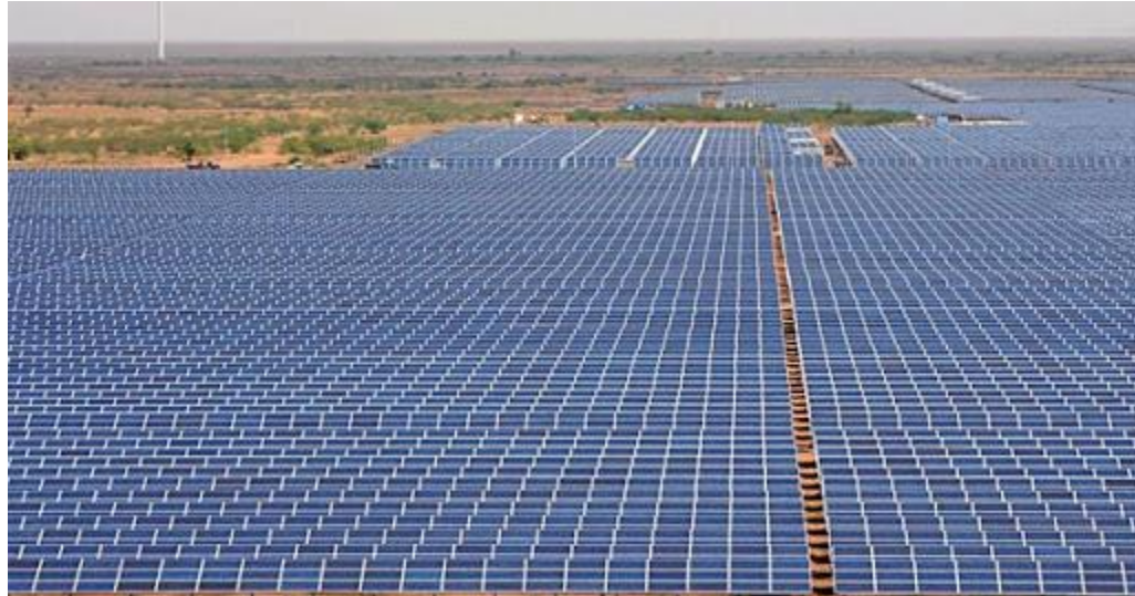
Figure 8.6 A large solar panel installation. Image from walkthroughindia.com
